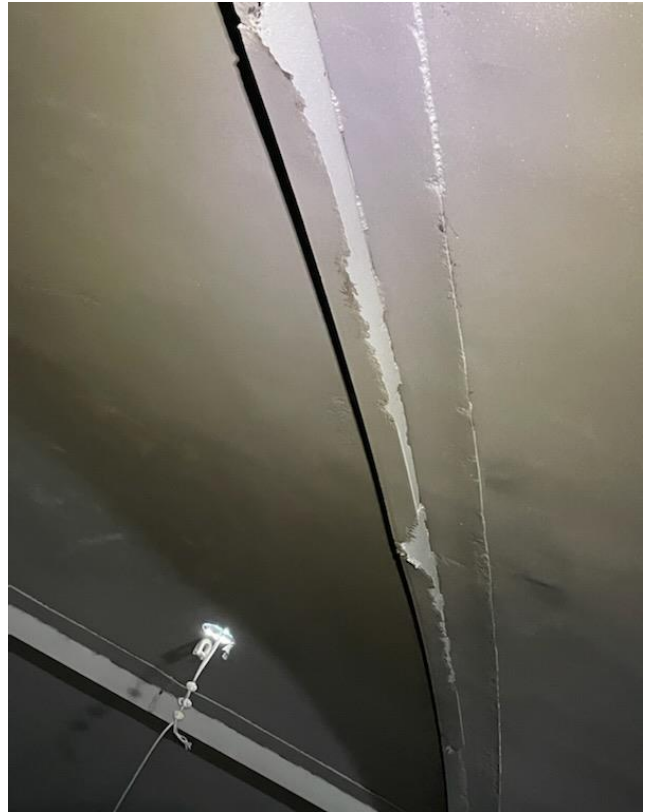
Corrosion on rafter
