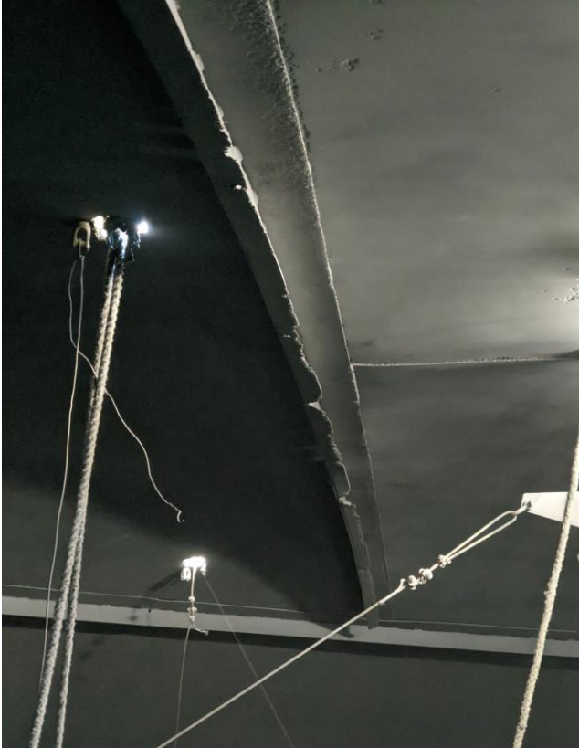
Corrosion on rafter
