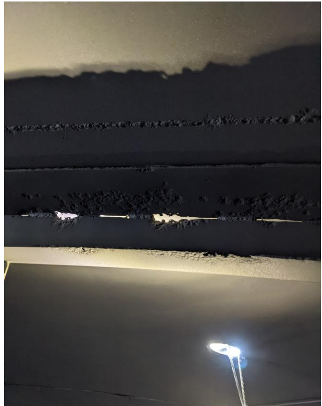
Corrosion through rafter, pitting on ceiling
