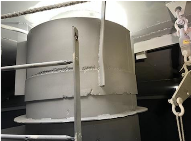
Corrosion on ring and dry riser tube
