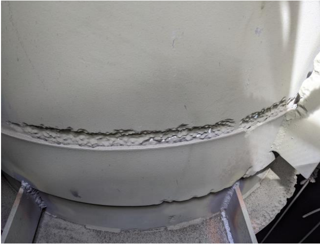
Pitting and pinholes above ring
