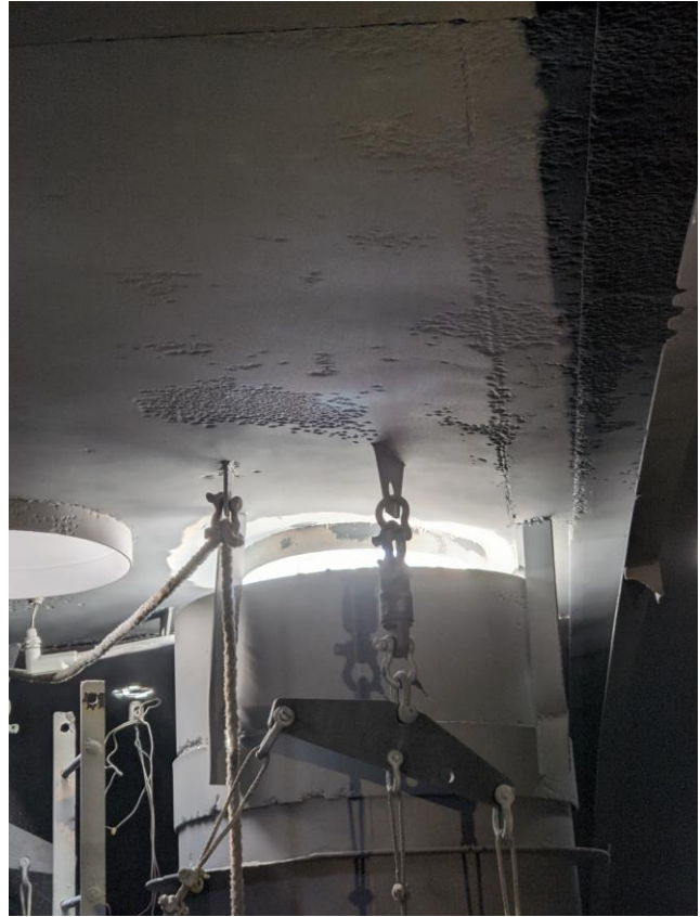
Corrosion on ring and tube, pitting on ceiling
