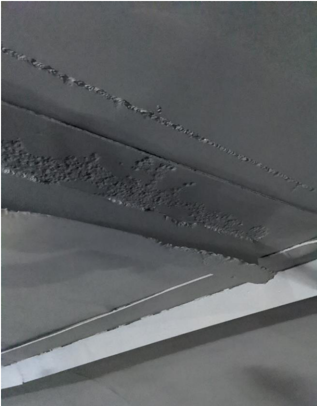
Pitting on ceiling, corrosion on rafter
