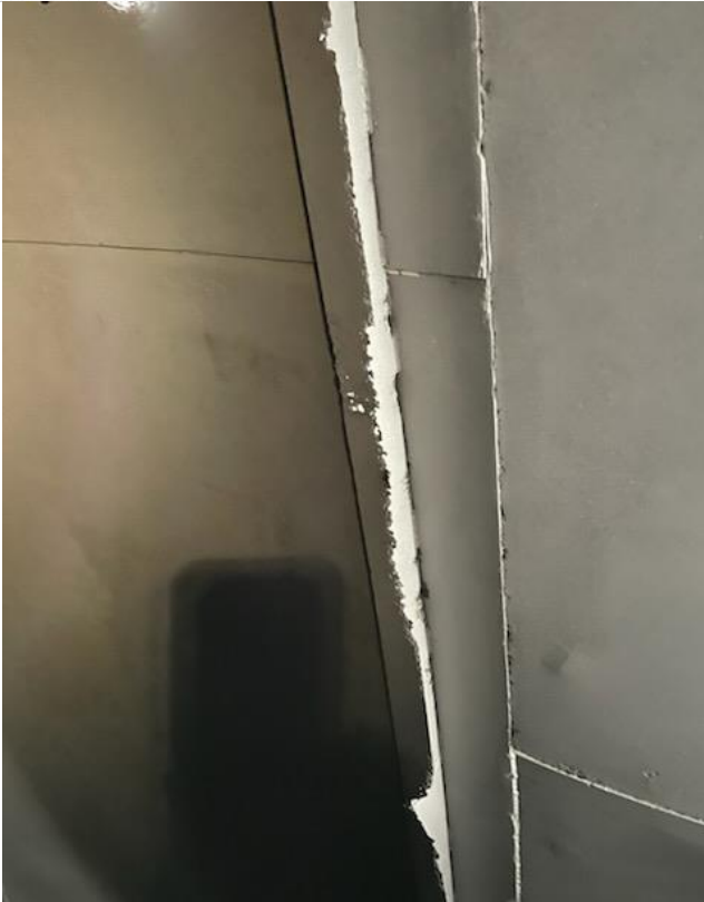
Corrosion on rafter
